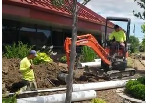
Drainage improvement construction. Source: How Much Slope When Installing a Commercial Underground Drainage System (frenchdrainman.com)
