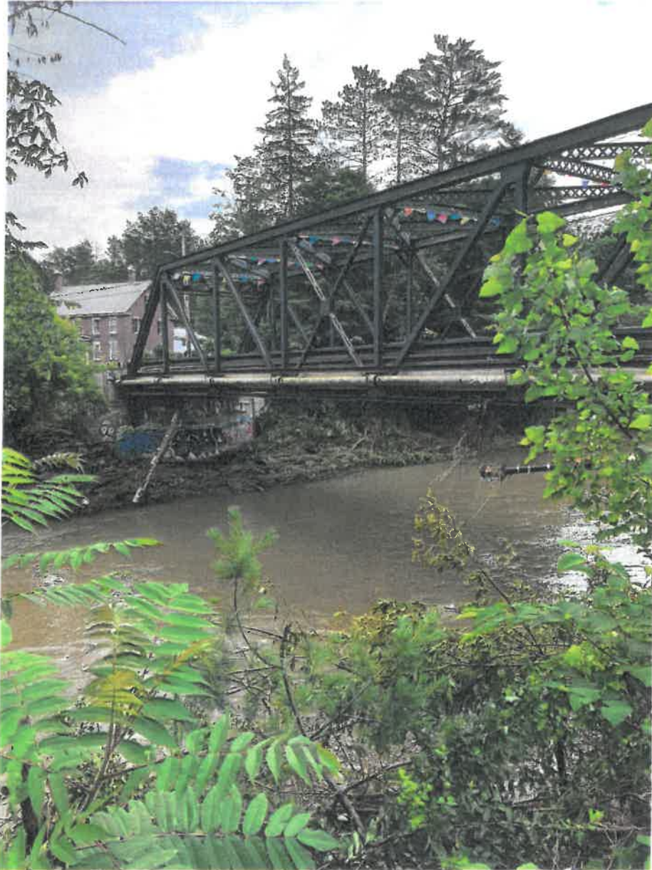
29- Railroad Street Bridge Severed 8" DI Sewer Crossing
