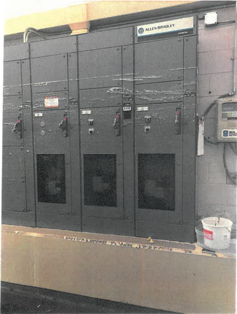
1 - High Water Mark on MCC
