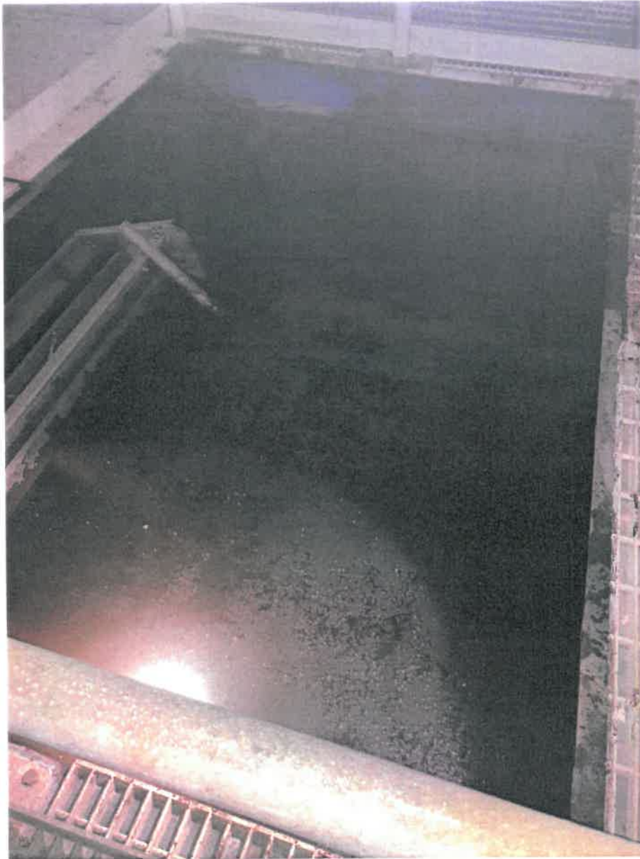
18- Sequencing Batch Reactor (SBR) Chamber with Decanter
