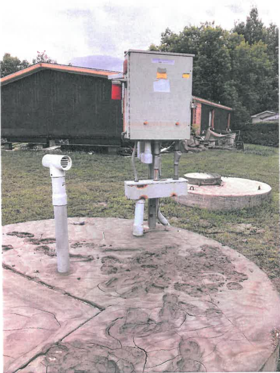
26- Highland Heights Pump Station
