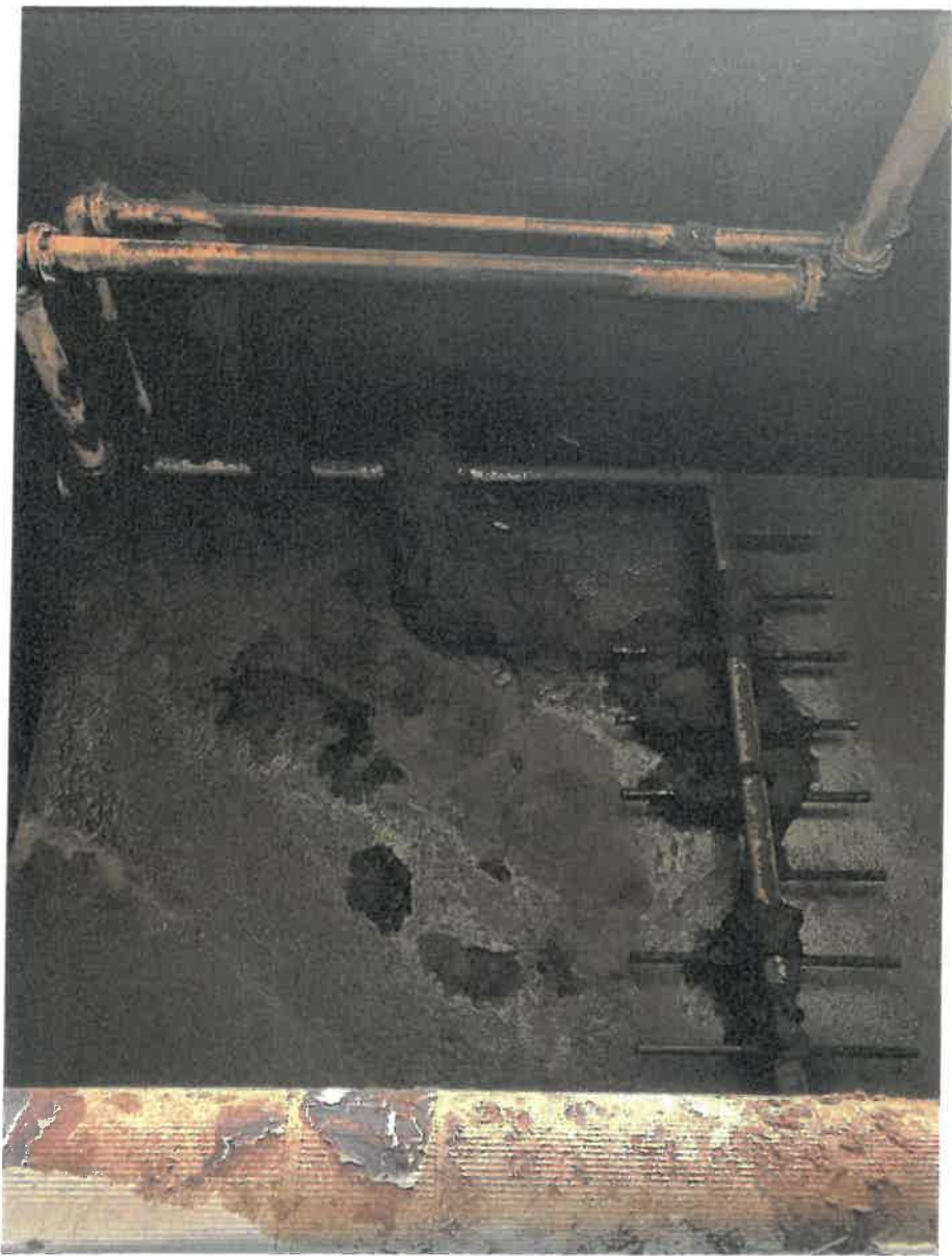
19- SBR Chamber After Pumping Out Flood Waters
