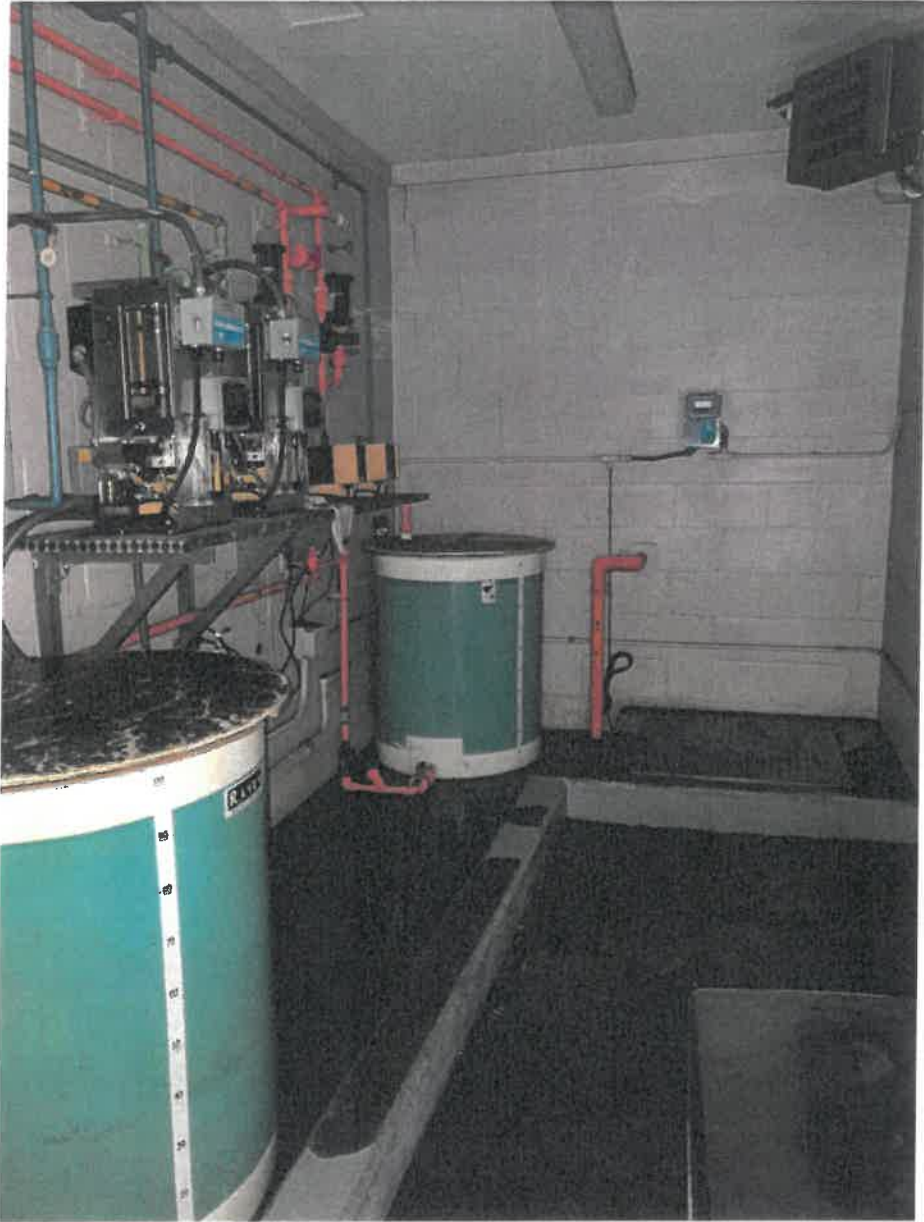
11- Chemical Feed Room with Tanks and Pumps
