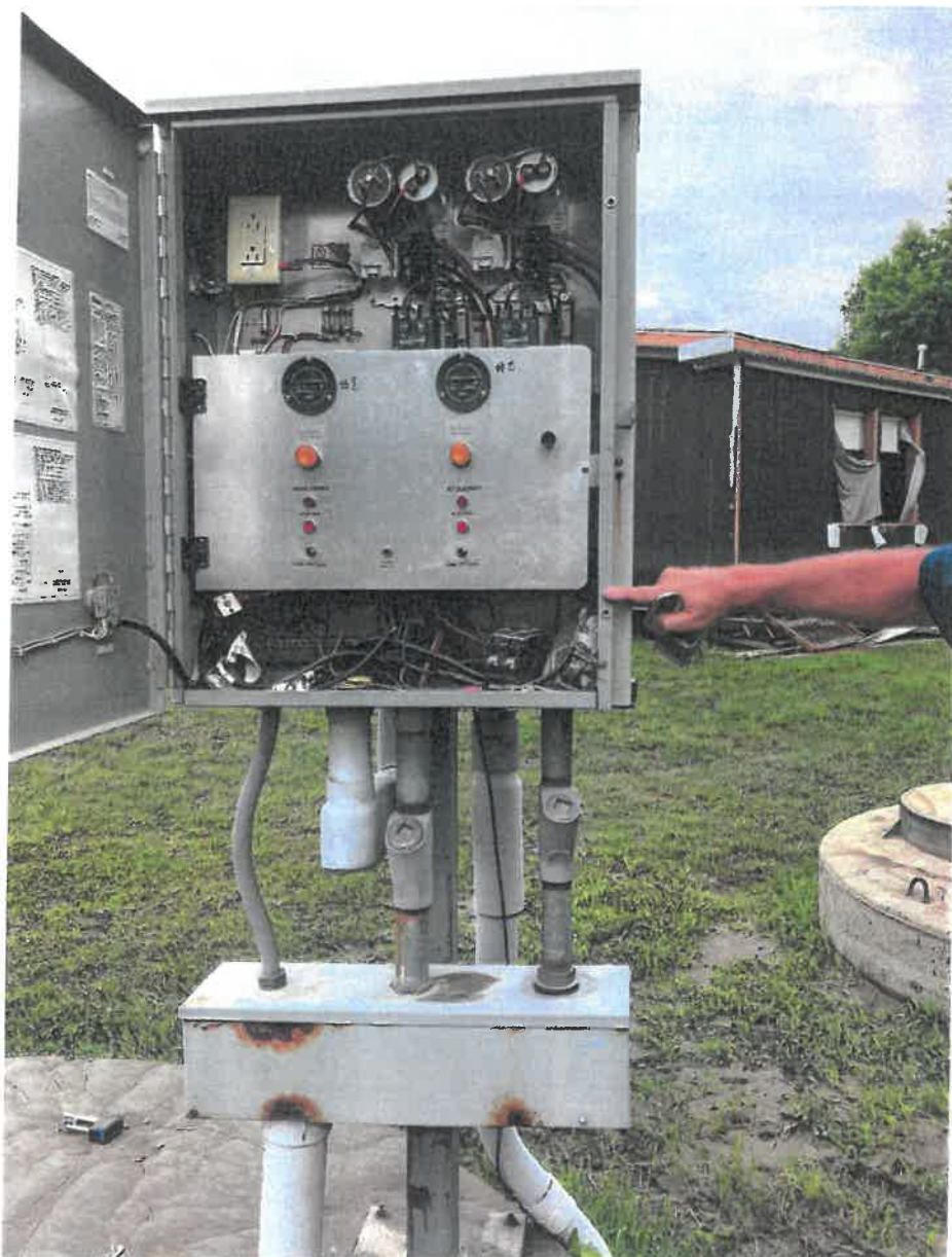
27- Highland Heights Pump Station Control Panel High Water Mark
