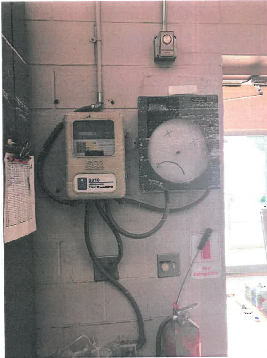
4- High Water Mark on Flow Meter and Chart Recorder
