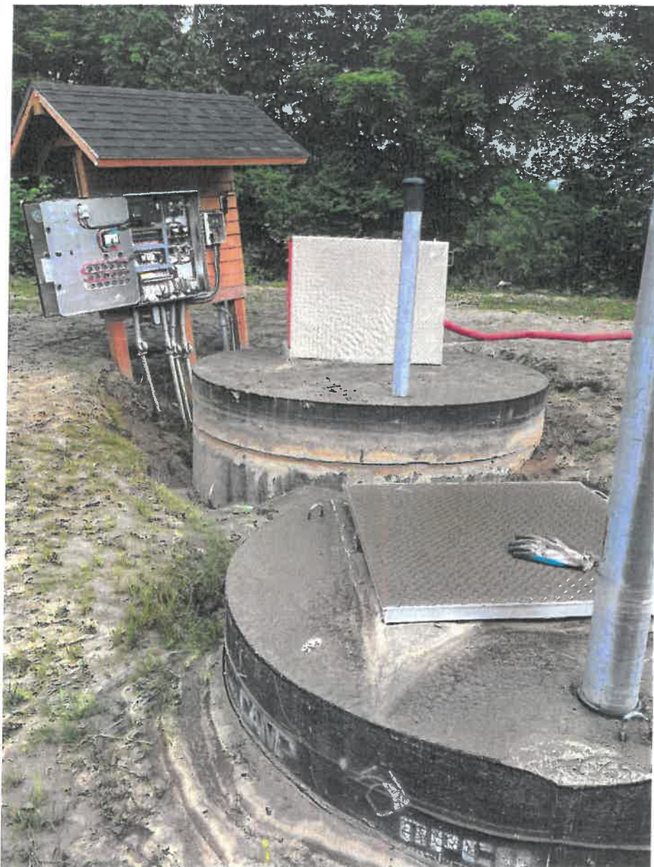
23- River Road West Pump Station
