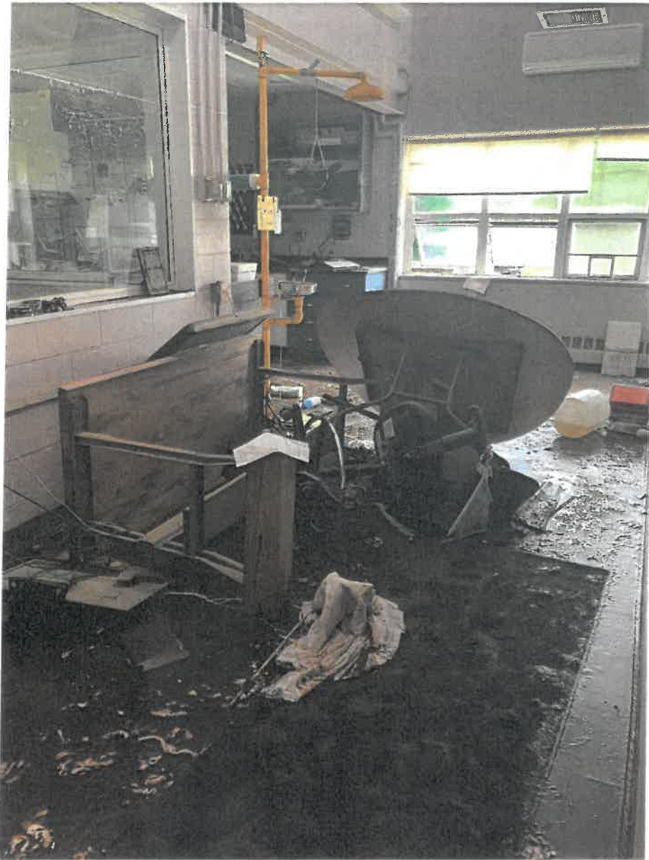
3- Post Flood Debris in Control Room
