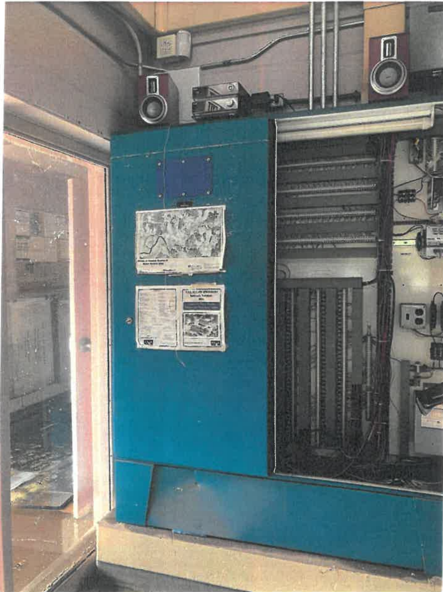
5- High Water Mark on Programmable Logic Controller (PLC) Cabinet
