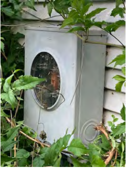
Missing electric meter
