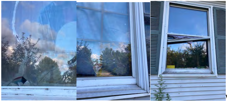
Various broken windows
